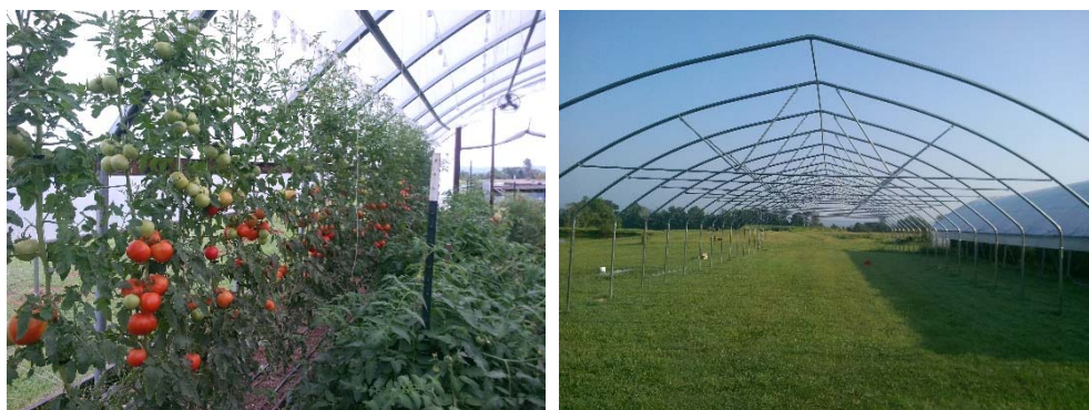
Left: Tomatoes in the DSAC high tunnel. Right: Our new high tunnel under construction.
