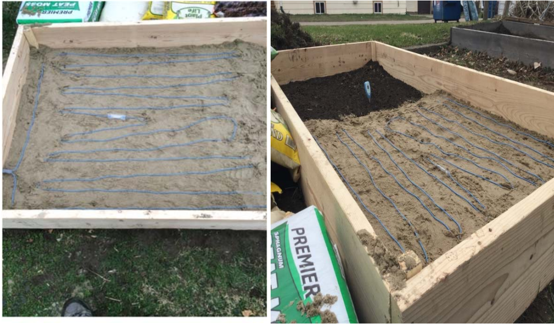
Soil heating cable on a 2-inch layer of sand
