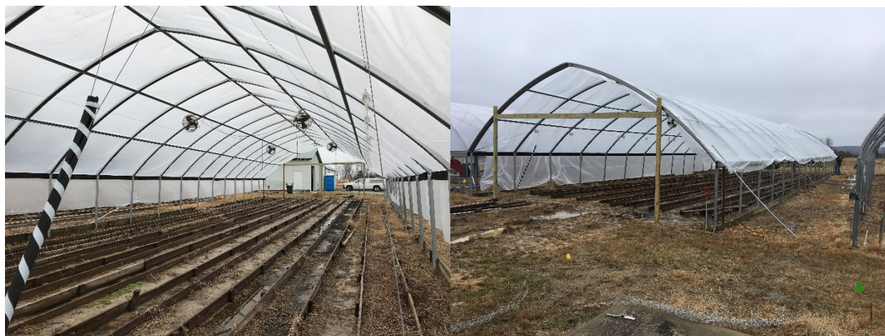
New cover and end wall structures on one of the high tunnels at the Dixon Springs Ag Center. Photos: B. Aly (left); N. Johanning (right)
